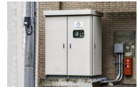
High-Voltage Power Services
